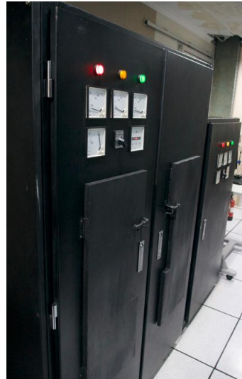
UPS (Uninterruptible Power Supply)
