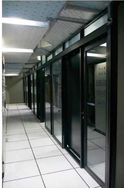
Fasilitas Data center TIFA 2
