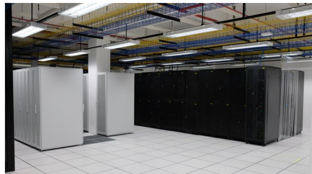
Fasilitas Data Center
