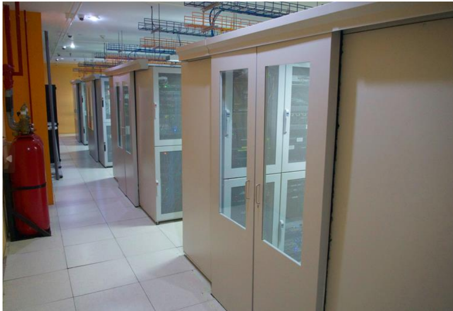
Fasilitas Data center
